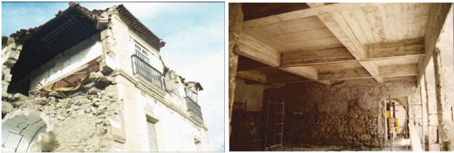
Fig. 9.4 Açores 1980 earthquake: damage to the monumental structures and reconstruction with reinforced concrete
