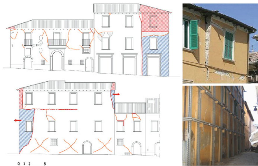
Fig. 20.26 Damage state in the building in Piazza della Prefettura: elevations and pictures
