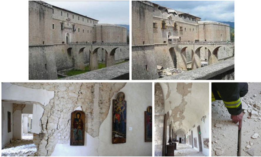
Fig. 20.16 Above: view of the L'Aquila castle (Spanish fortress) before and after the earthquake; below: severe damage recorded in the internal area of the S-East wing
