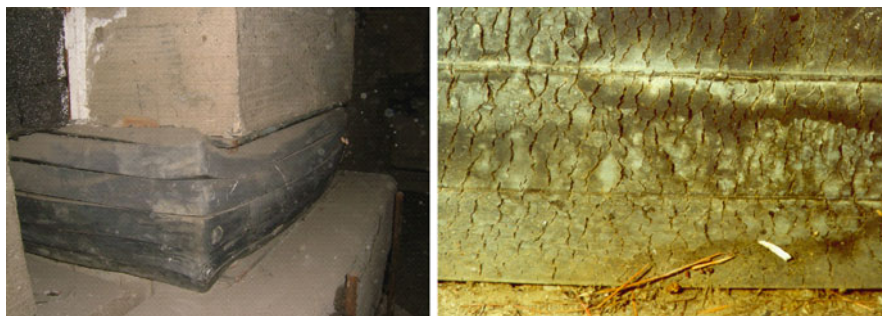
Fig. 17.2 Smashed and cracked old bearings
