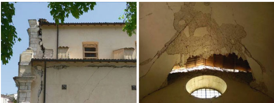
Fig. 20.2 Incipient out-of-plane overturning of the façade, church of Santa Gemma in Goriano Sicolli ( left ); collapsed vault, church of Santa Maria del Soccorso in L'Aquila ( right )
