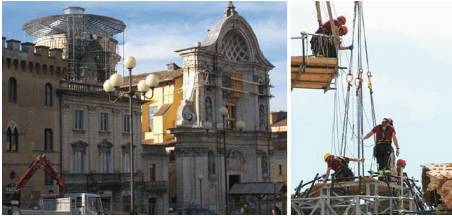
Fig. 20.5 Drum of the Anime Sante's church in the historical centre of L'Aquila ( left ); special groups of National Fire Brigade men at work on the Anime Sante's dome ( right )
