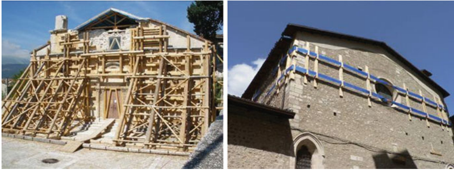
Fig. 20.6 Propping of the façade of Santa Giusta church in Bazzano ( left ). Polyester bands on the façade of San Giuseppe dei Minimi's church in the historical centre of L'Aquila ( right )
