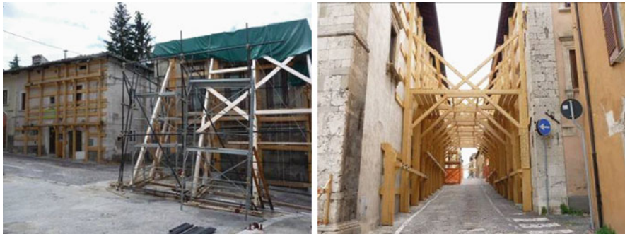
Fig. 20.9 Three types of safety measures on façades in the historic centre of L'Aquila: wooden grids and ties, traditional props, shoring systems acting on facing buildings
