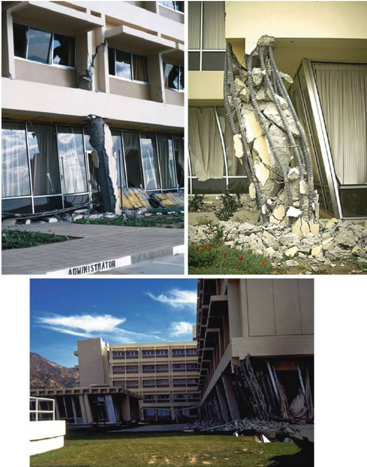
Fig. 10.6 Damage at the Olive View UCLA hospital, San Fernando earthquake (1971, photo USGS). Note the different response of columns with rectangular and spiral confinement, the shear collapse at the first floor and the relative displacement at the ground floor, estimated in 81 cm
